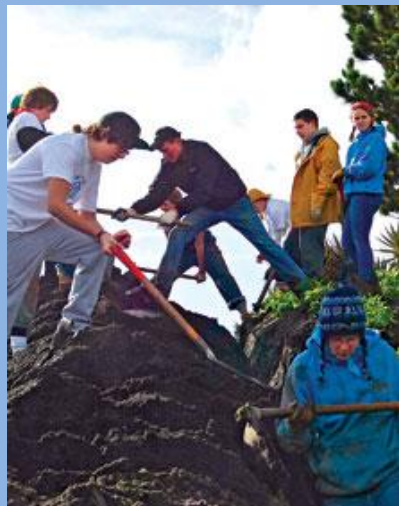
Top: Tony Riggio, a member of the Rotary Club of Westport, Connecticut, USA. Bottom: Rotarians work with young people in the Builders Beyond Borders program to install pipes that will carry water to the mountain town.
